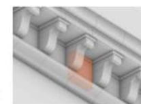
Frieze Panel 10/71 cracked 0/71 spalled 0/71 missing
