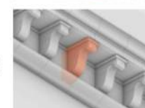
Corbel 41/77 cracked 21/77 spalled 0/77 missing 47/77 steel brace applied
