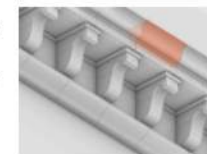
Cornice Cap 36/79 cracked 14/79 spalled 1/79 missing
