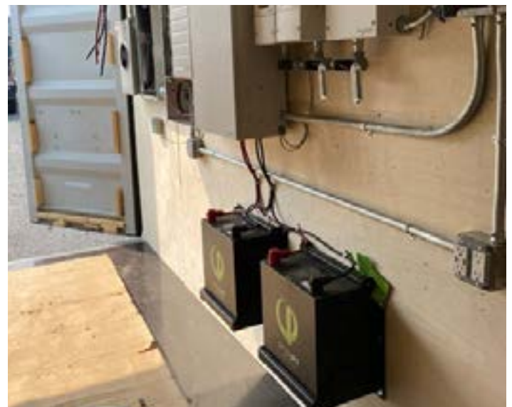
City Tech CSC Solar+Storage Training Lab, BNYDC
